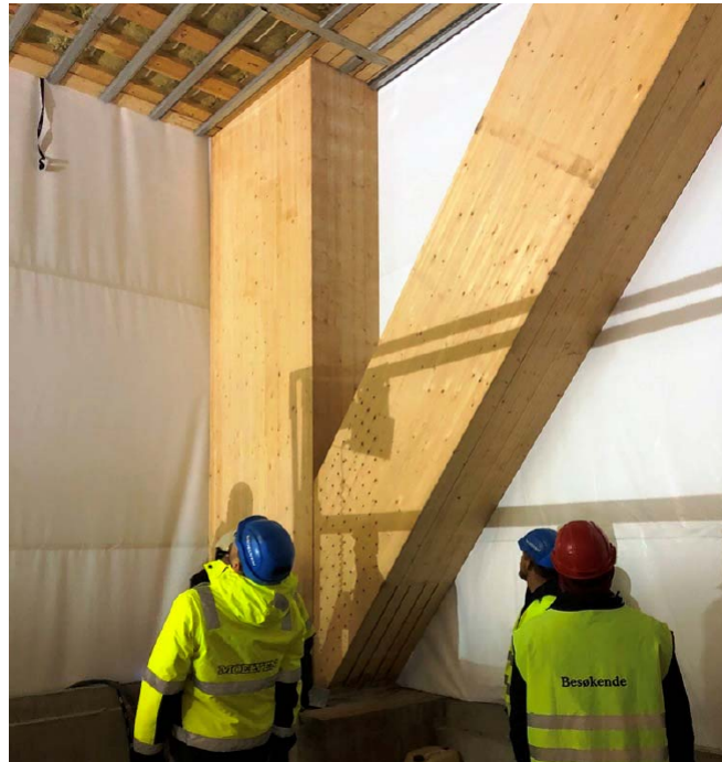
Figure 1.2: Images of the massive slotted-in steel plate timber connections used within the Mjøsa Tower. Source: Images from the presentation by CEO of Moelven Limtre, Rune Abrahamsen, at the Internationales Holzbau-Forum IHF in 2017
